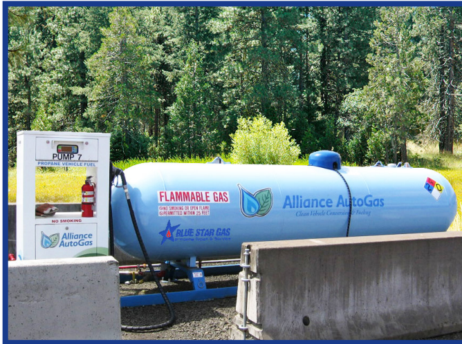
Polk County Sheriff's Office on-site fueling infrastructure
